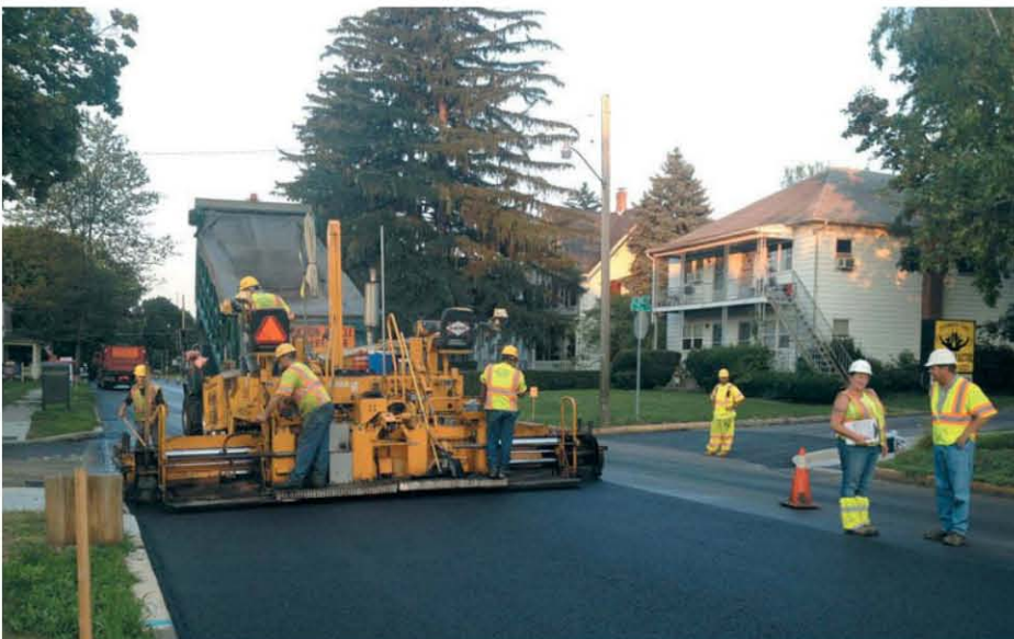
Pennsylvania State Route 45 served as one of the test beds for fiber-reinforced asphalt.
