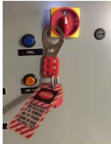
Figure 10: Locking-out the disconnect on the main control panel.
