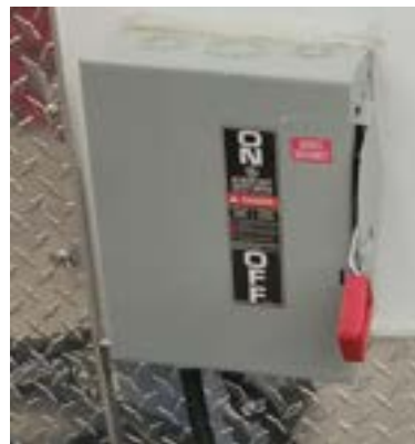
Figure 3: The electrical disconnect enclosure.
