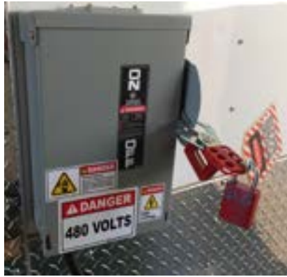
Figure 14: Lock-out/tag-out of the electrical disconnect enclosure (mobile system).
