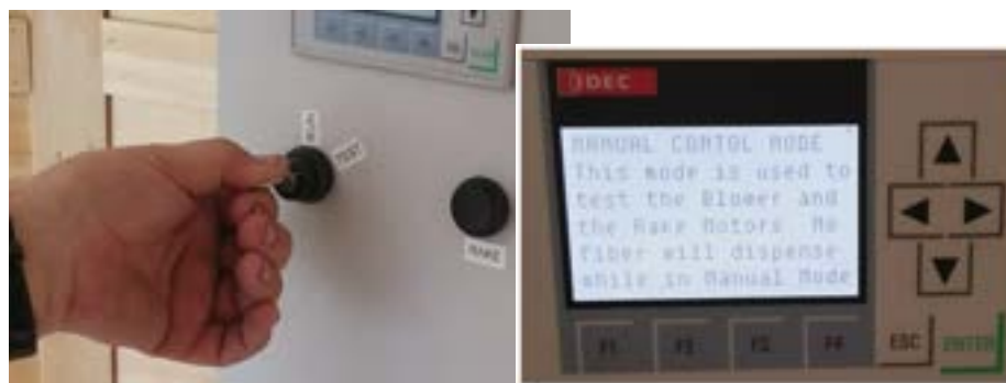
Figure 11: System in Manual control mode.
