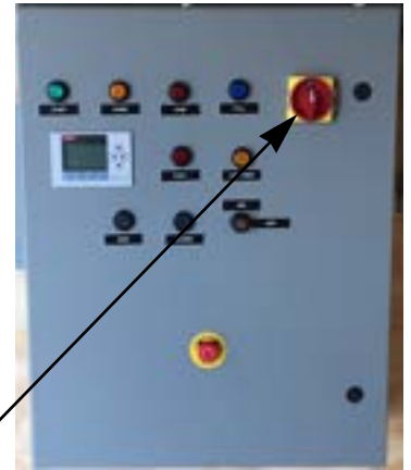
Main control panel
