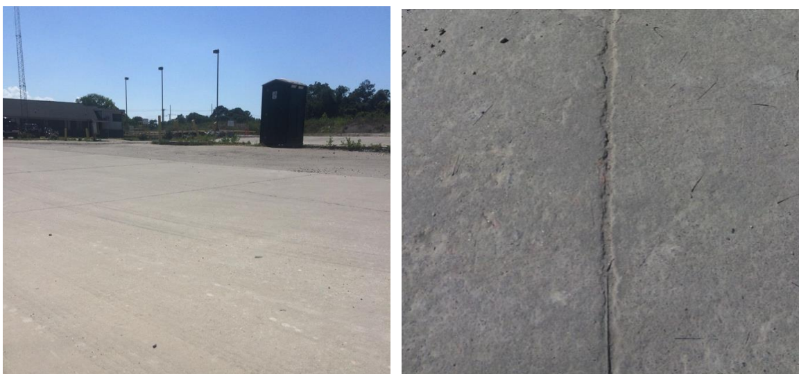
Figure 6. Pavement Condition after 8 Years
